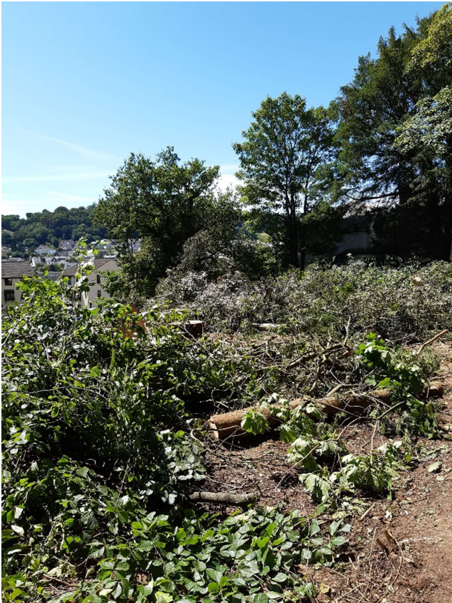
View of T3 Sycamore ,TIYew and T2 Sycamore from within the site located to the right of the photo in July 2020
